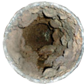
Inside of a corroded metal pipe
